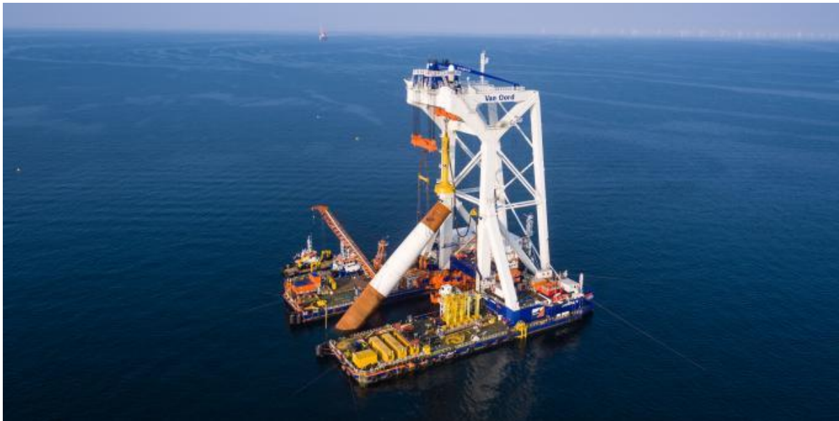
Figure 4.1 The Svanen, upending a monopile at the Kriegers Flak wind farm 2020 (Van Oord, 2020)
