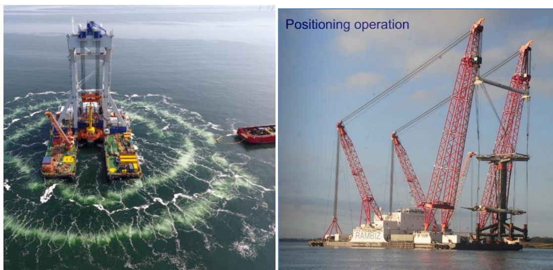
Figure 2.1.4: Left: Van Oord's Heavy lift vessel Svanen [source ("Vesselfinder.com," 2020)]. Right: Rambiz positioning the SeaGen at Strangford narrows (Ireland), at a water depth of 25m +/-2m, on a jacket foundation (Fraenkel, 2009).
